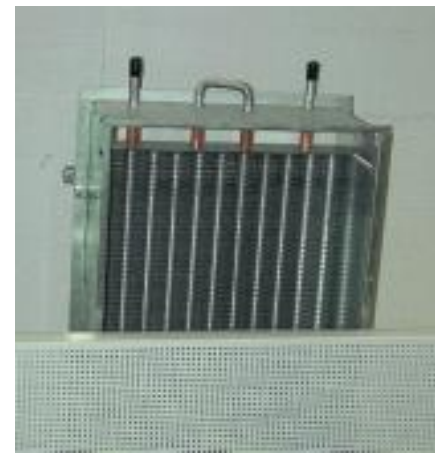
Fig. 3: Concealed chilled beam installation above a perforated false ceiling
