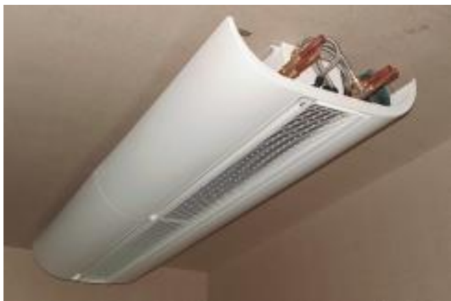
Fig. 14: Active chilled beam with "wings" concealing ceiling utilities
