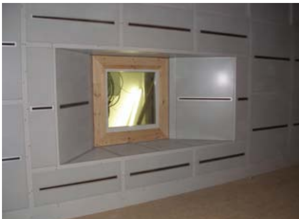
Supply air wall with perforated metal sheet panels and slot diffusers. Window for the supervision of the shooter with air distributing perforated metal sheet panels.
