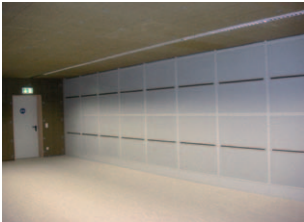
Supply air wall with perforated metal sheet panels and slot diffusers
