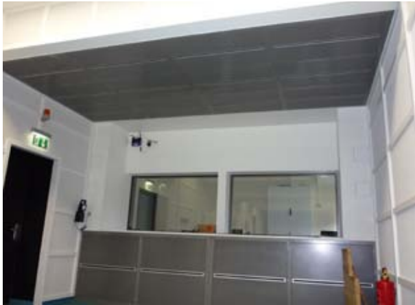
Indoor firing range with supply air ceiling and wall
