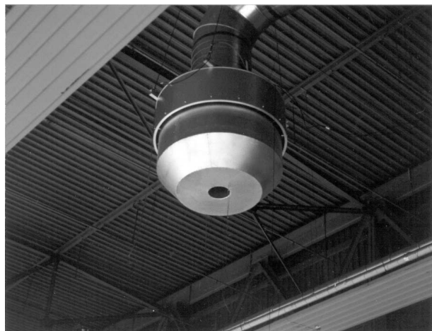
Fig. 2: Conical displacement outlet on the ceiling of a 26 m high hall
