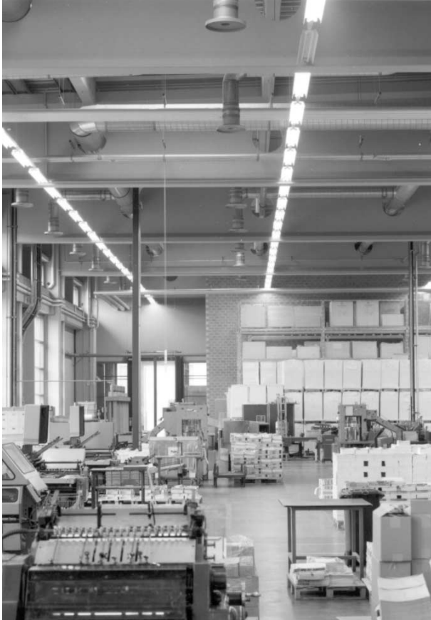
Fig. 9: Radial displacement outlet in a printing shop
