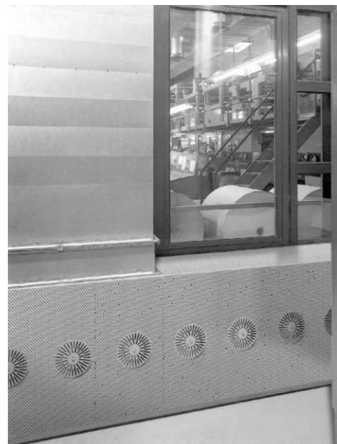
Figure 8: Air outlet in a printing hall
