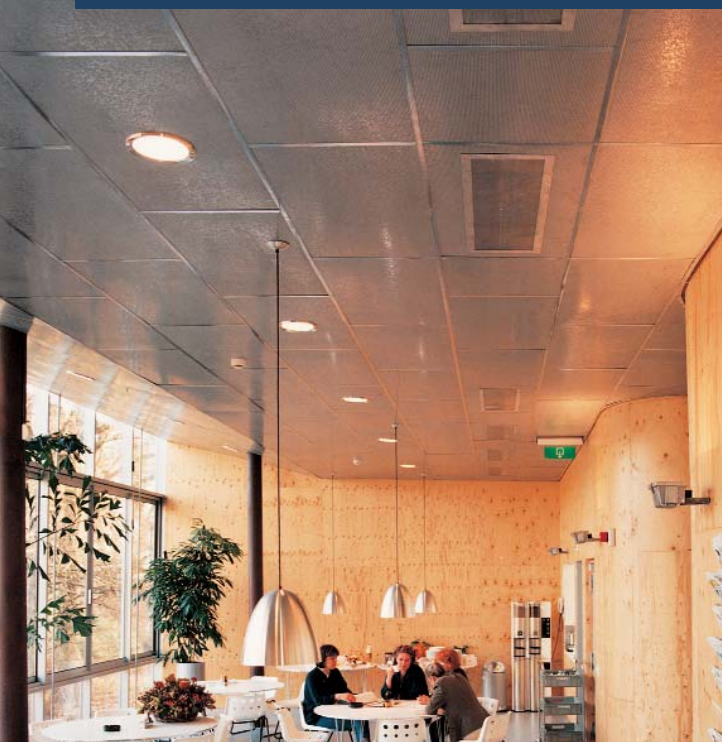
Ceiling displacement outlet, type Q-DN, in the cafeteria at 'Mediapark Hilversum', Hilversum / NL
