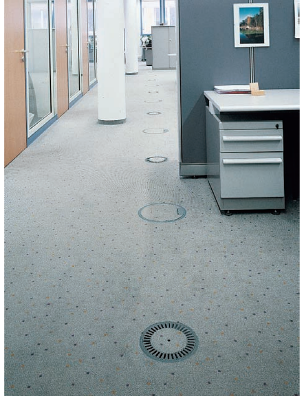
Figure 5: NTK floor twist outlet in an office building
