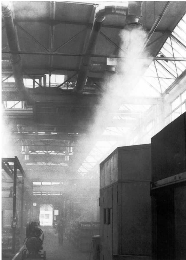
Jet spread in heating mode made visible with smoke tracer: The warm, vertical supply air jets penetrate deep into the occupied zone.
