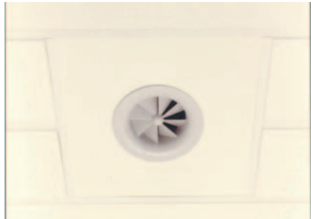
Twist outlet installed in a closed false ceiling
