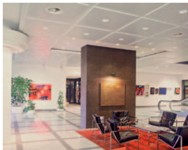
Twist outlet in the entrance hall of DEA Mineralöl AG, Hamburg / D
